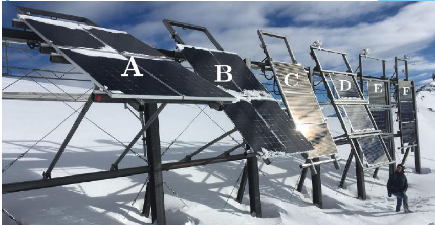
Total Installation (EKZ+ ZHAW)
